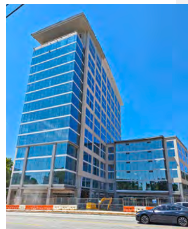
(left) The Marcus Center for Advanced Rehabilitation building on Shepherd's main campus is "topped out." (right) The Arthur M. Blank Family Residences tower at 1860 Peachtree Road is nearing completion.
